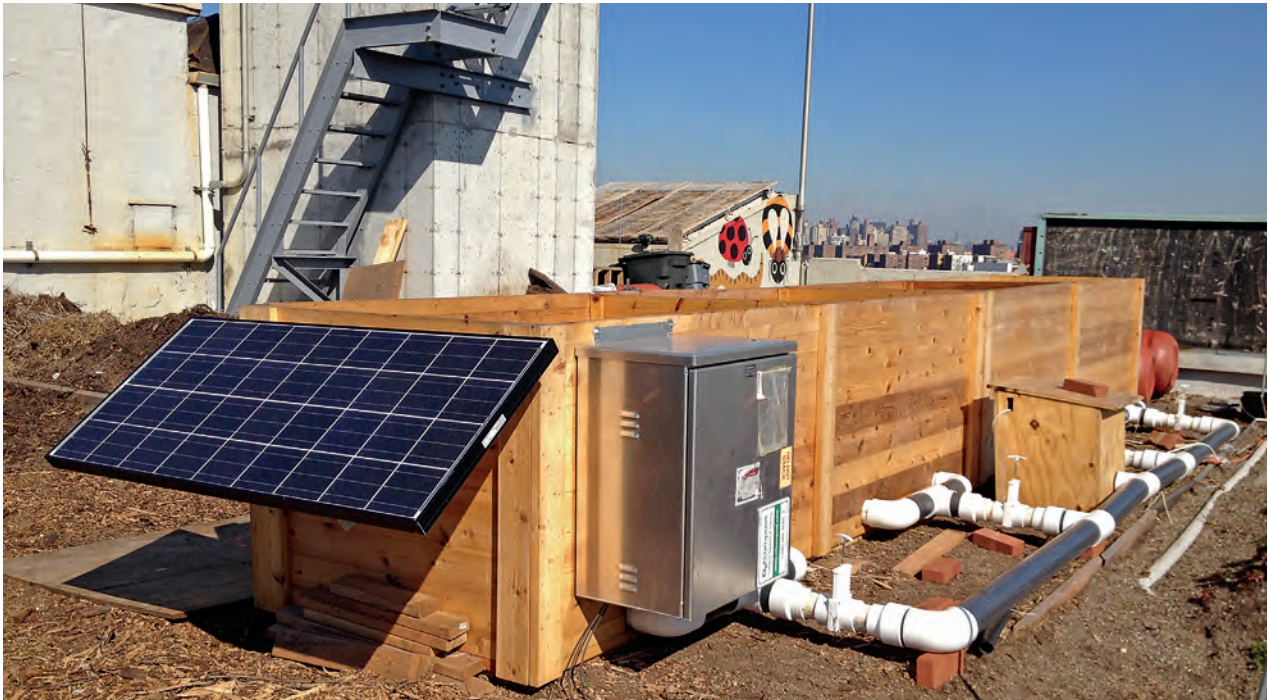
Solar powered forced aeration system in wood bins built by the NYC Compost Project Hosted by Big Reuse at Brooklyn Grange's rooftop farm in Long Island City.
