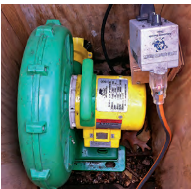
Fan used to blow air into perforated tubing.
